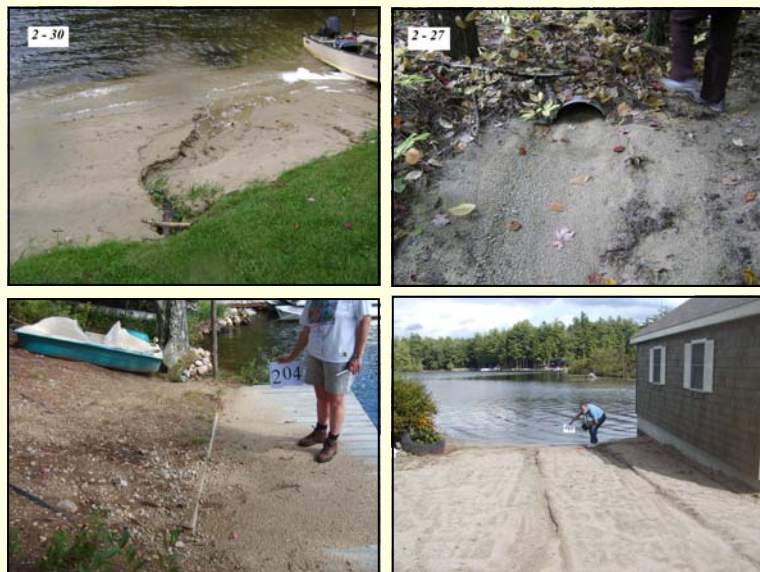
Examples of Identified Erosion Problems
